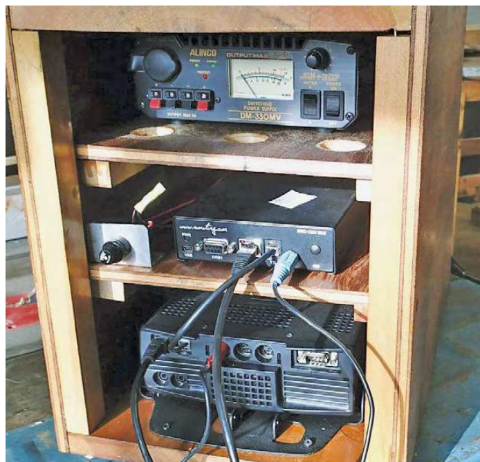
The front of the remote station in a box as it was being wired. Note the small fuse block to power the RRC box. From top to bottom: the 12 V power supply, RRC radio unit, and TS-480SAT transceiver in a mobile mount bracket. The top interior shelf shows the holes for flow-through cooling.
